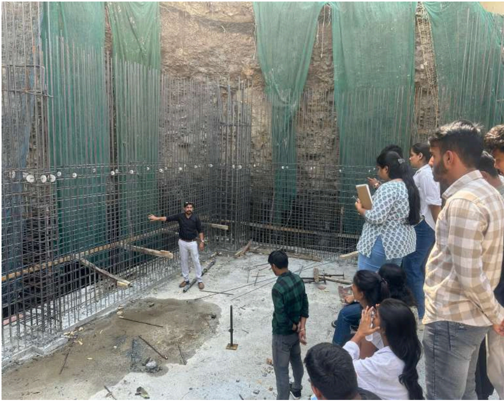
Site Visit: Bharati Vidyapeeth University Campus SY B.Arch students explored retaining wall materials, construction techniques, and failure analysis, enhancing their understanding of structural stability and site-specific design in Building Construction and Materials III on 2 September 2024.
