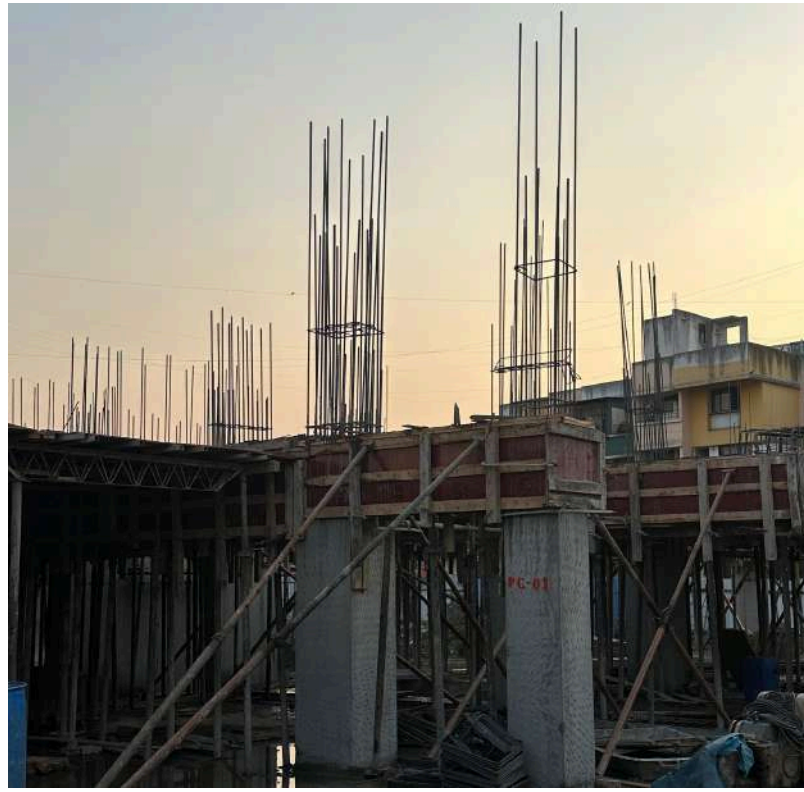
Site Visit - Shuttering Techniques - Second-year B.Arch students explored shuttering techniques at a residential project in Ambegaon on 11 th November 2024, gaining practical insights into materials, construction methods, and cost considerations.
